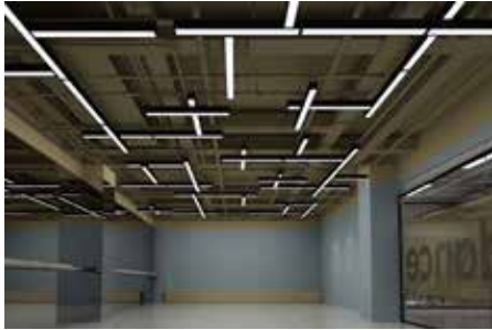
İç Mekan Aydınlatma Indoor Lighting
